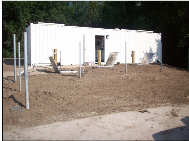
Brisbane Public School—Waterloo Biofilter Shipping Container
