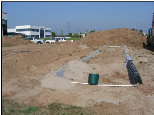
Shallow Buried Trench Disposal System
