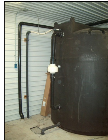
Polyethylene Tank in Building
