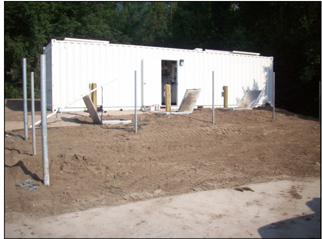
Brisbane Public School—Waterloo Biofilter Shipping Container
