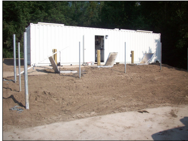
Brisbane Public School—Waterloo Biofilter Shipping Container
