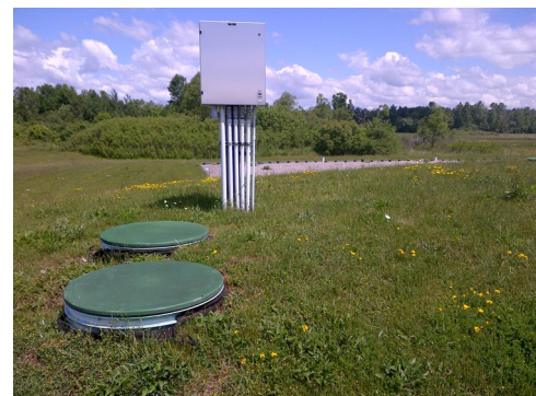
Existing Pump Tanks
