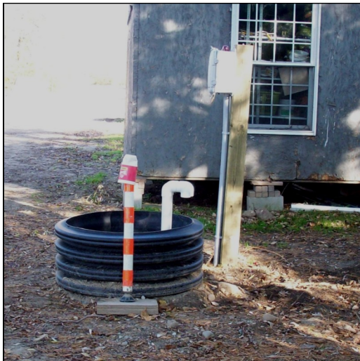
Final Installation of Pump Station and Control Panel
